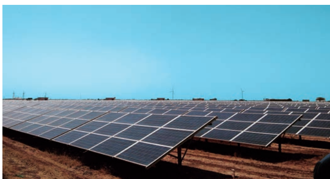
Solar power plant in Gujarat, India. © Prajapati Karan v/ Shutterstock
